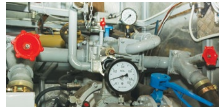
Pump and valve control
